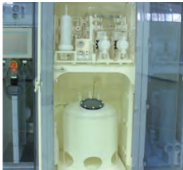
SIMONA® PVDF: Chemical mixing unit
